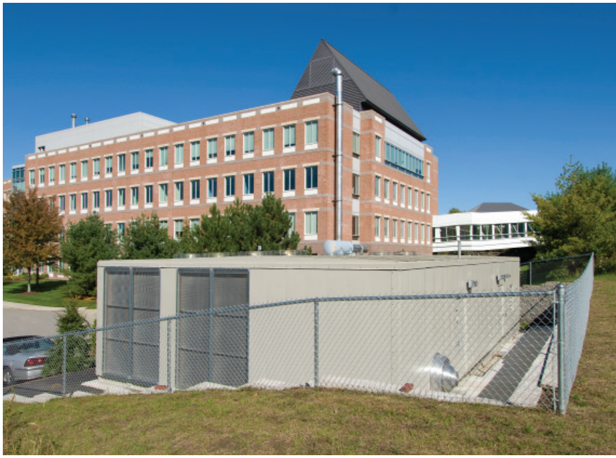
The Mammoth chiller plant installed at Avid provides a totally self-contained system, precommissioned for plug-and-play operation, sole source responsibility, portability if the facility is vacated, and it meets aesthetic requirements of the building owner.
