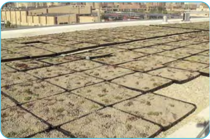
A "green" roof helps reduce building load during the day.
