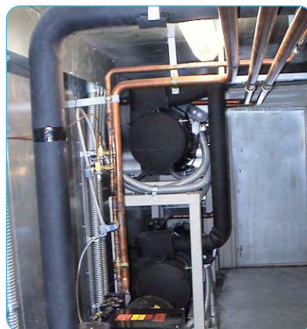
iPEC provides plenty of service space for Dx compressors and accessory maintenance. Co-locating equipment in a common location can save space and reduce maintenance costs.
