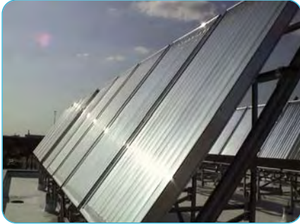
Roof-mounted solar collectors provide for most domestic hot water.
