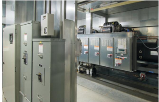
Chillers and Chiller Plants
