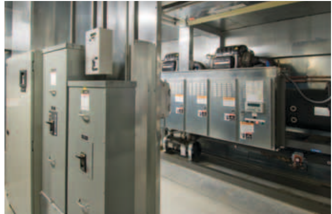
Chillers and Chiller Plants
